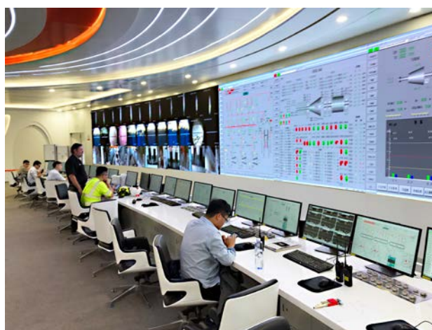
Modern control room at Shenzhen East.
